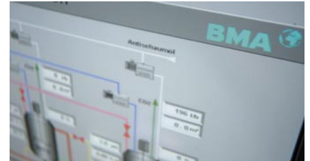
PLC user surface of the Lentikat pilot plant
